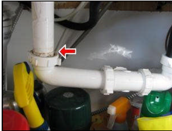
6.0 Picture 1 Missing "P" trap
