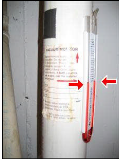
6.4 Picture 2 Mitigation system inoperative
