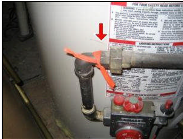
6.4 Picture 1 Gas leak
