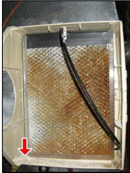
8.3 Picture 1 Filter needs replacement
