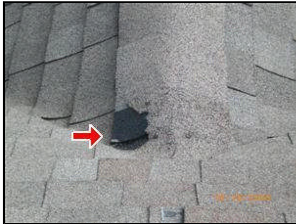
1.0 Picture 1 Broken shingle
