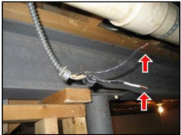
7.3 Picture 1 Open wiring
