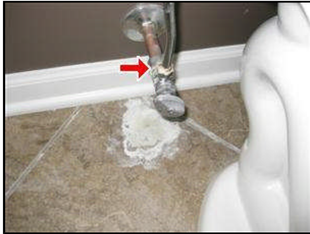
6.1 Picture 1 Leaky valve
