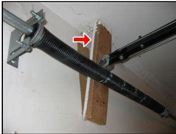
3.0 Picture 1 Support needs to be secured
