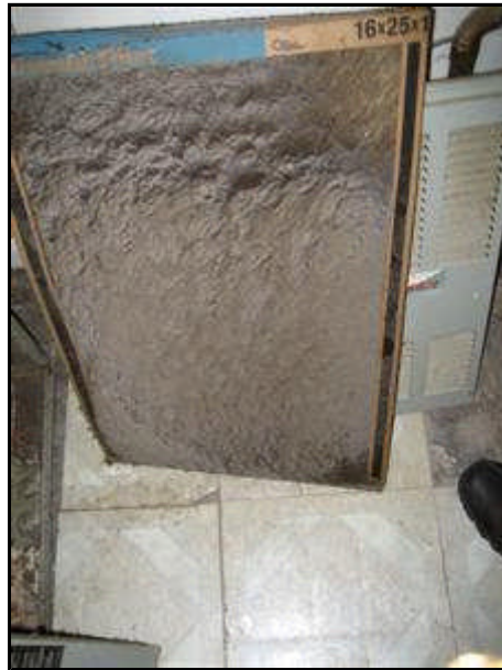
8.3 Picture 2 Plugged filter
