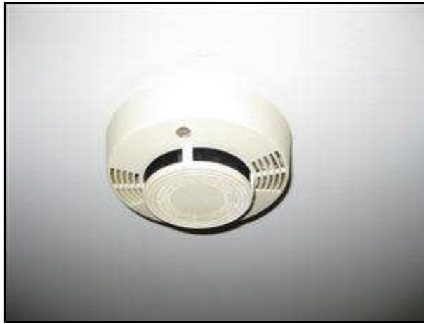
7.7 Picture 1 Needs replacement
